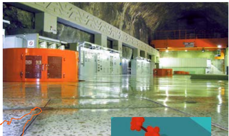
Unit hall, San Carlos hydropower station
