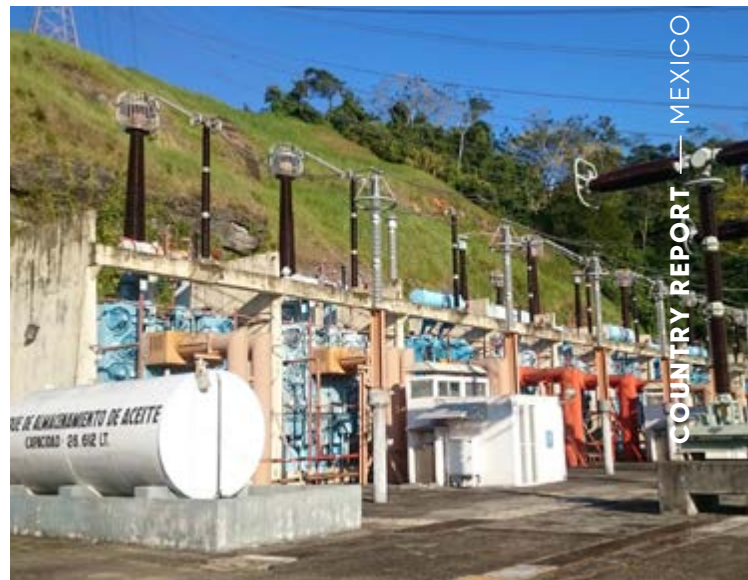
Main transformers, Malpaso hydropower plant
