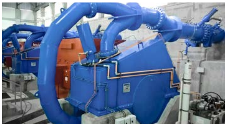
Unit hall, Sigchos hydropower plant
