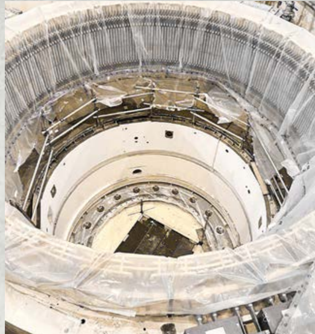
Good practice – Stator protection
