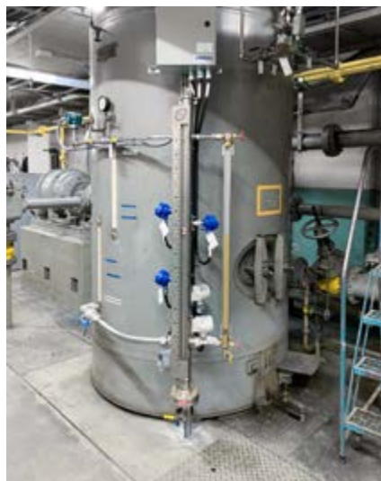
Accumulator instrumentation at the Des Joachims hydropower plant
