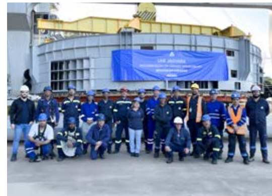
Installation team of the rehabilitation of the generator of Unit 1 at Jaguara hydropower plant
