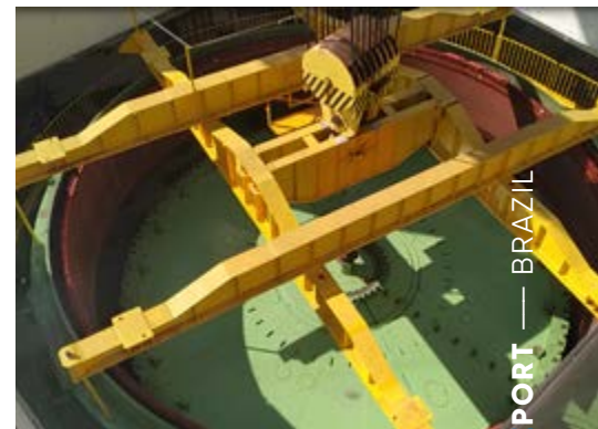
Generator of Unit 1 in the pit of Jaguara hydropower plant on the Rio Grande
