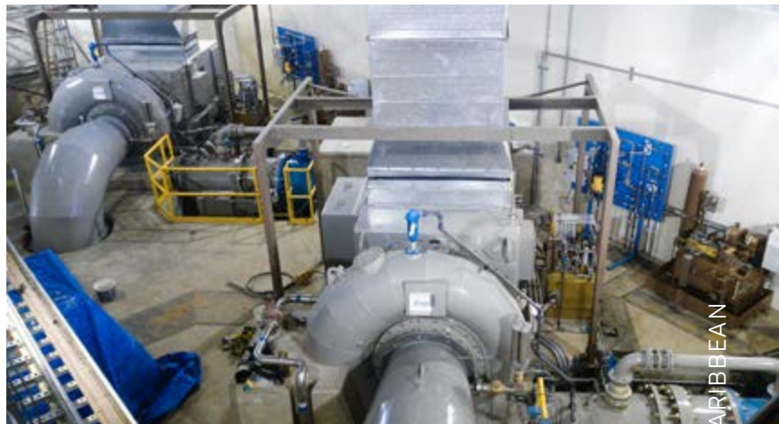
Unit hall at Maggotty hydropower plant, Jamaica
