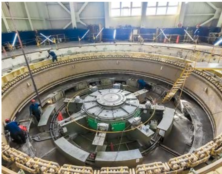
Combined bearing, Unit 1, La Villita hydropower plant
