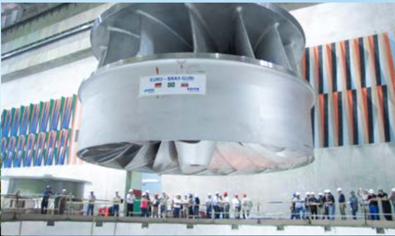
Installation of one of the world's largest Francis runners (770 MW) in Simón Bolívar 'Guri' hydroelectric power plant in 2012.
