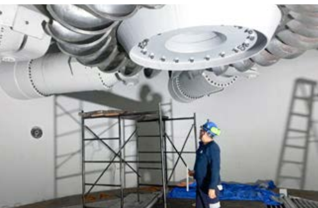
Pelton runner at Zimapan hydropower plant
