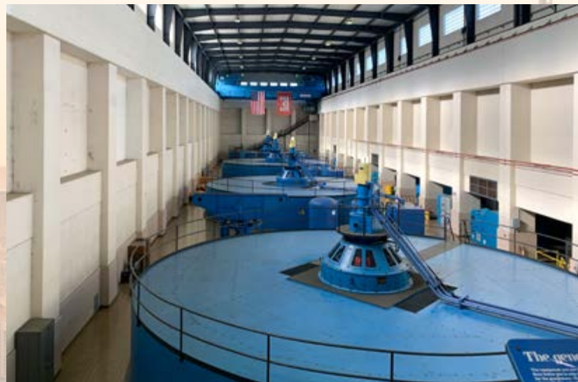
Unit hall, Barkley hydropower station
