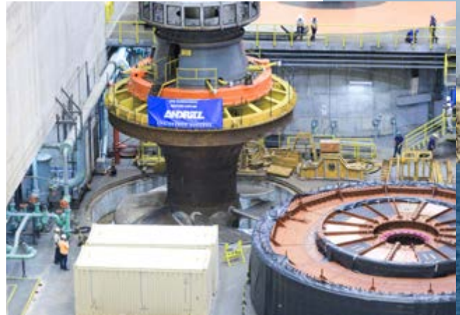
Outside view (right) and installation work of Kaplan turbine (above) at Sobradinho hydropower plant on the São Francisco River, Brazil
