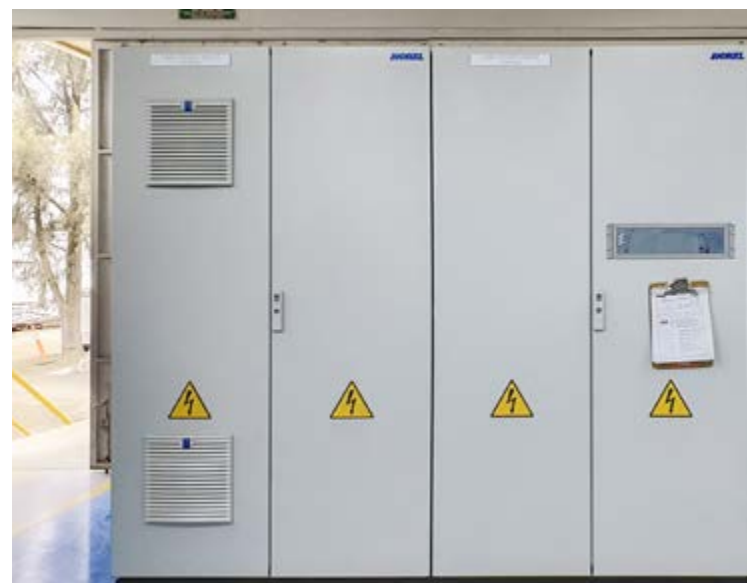
Electric cubicles at Mazatepec hydropower plant
