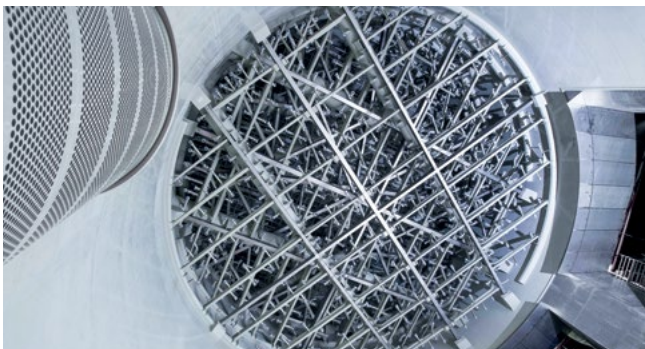
Scrubber at Neurath Power Plant, Germany
