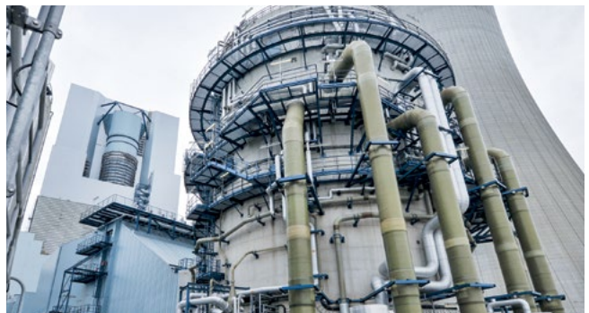
World's largest absorber in Neurath, Germany
