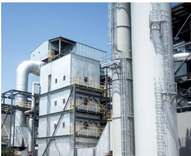
Dry Sorbent Injection and Tail-End SCR, Conyers (GA), Pratt, USA
