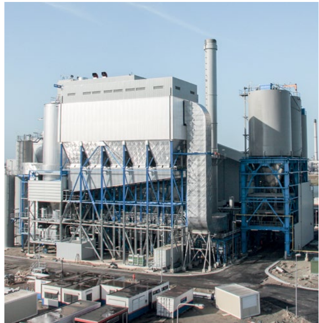
TurboSorp, Fabric Filter, SCR, Moerdijk, Netherlands
