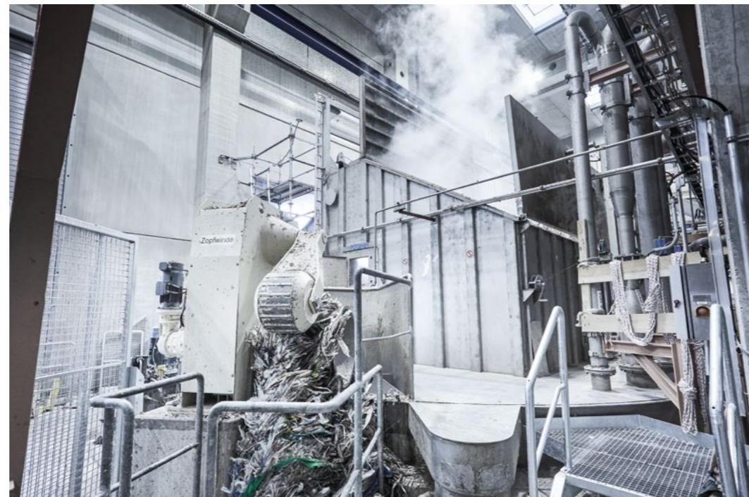
The pulping system with detashing includes a 130 m³ FibreSolve FSR pulper – the largest LC pulper ANDRITZ ever installed in Europe.
