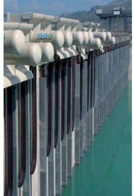
Turbine-generator units in maintenance position
