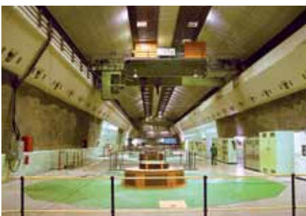
t Underground powerhouse
