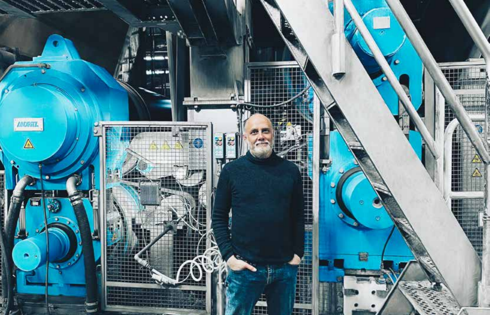
The new PrimePress X shoe press at Merati's BM1 (Italy) is operating at a line load of 2,000 kN/m – a world record! It enables Merati to achieve extraordinary dry contents of up to 59%. In addition, the runability of the machine increased and the specific energy consumption decreased significantly. Photo: Marco Merati, Managing Director, A. Merati & C. Cartiera di Laveno
