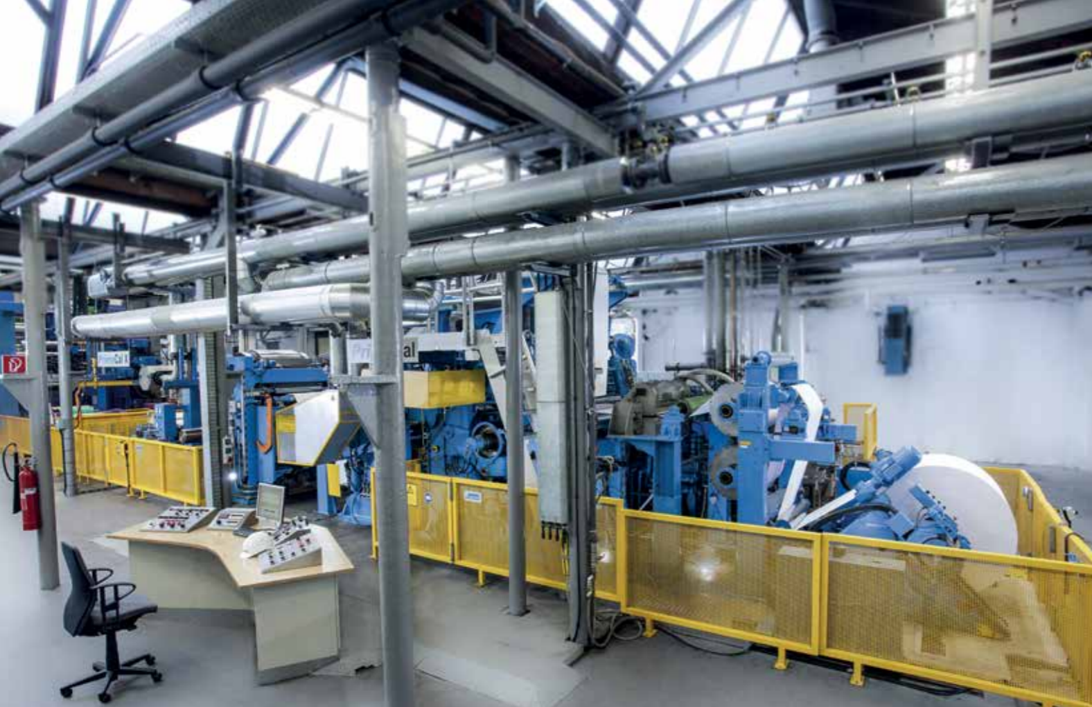
At the Paper Technology Center in Krefeld, Germany, you can choose between our PrimeCal Hard/Soft calender, PrimeCal X shoe calender, and PrimeCal Y belt calender, which can be configured in many ways to take papermaking to a new level. The pilot plant is available for running trials of printing/writing papers, special papers, cartonboard, and packaging grades with its 2x2 or 8+5 rolls and a maximum speed of 1,500 m/min at a surface temperature up to 220° C.
