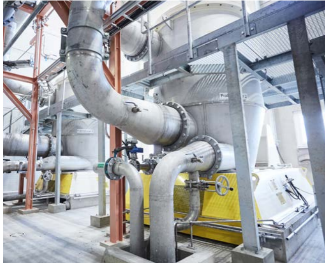
The fractionation section comprises a combination of existing equipment and a ModuScreen A with a matched screen basket/rotor concept.
