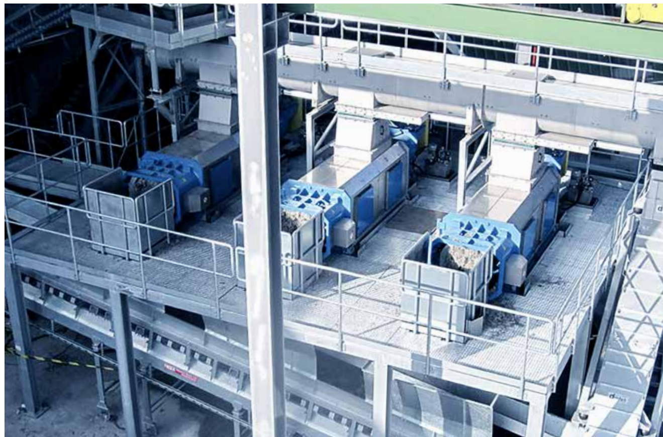
Three parallel Reject Compactor ReCo-C units
